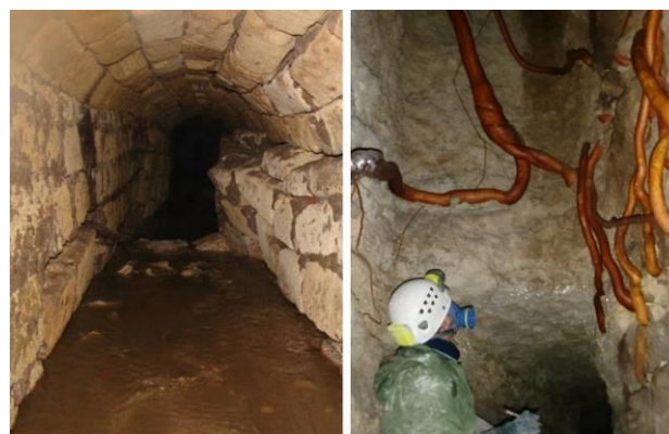
Figure 16. Deterioration due to sidewall collapse and degradation due to root action (Photographic archives CAI Palermo Speleological Group).
