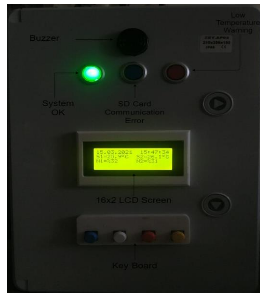
Figure 2.3. The front surface of the electrical panel.
