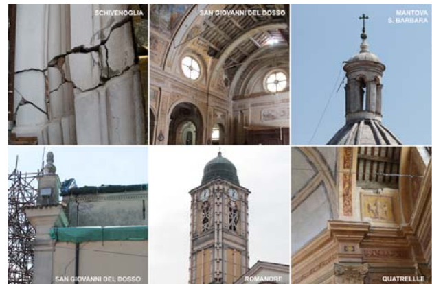
Figure 1: some photos of different damages in the churches of Diocese of Mantua
