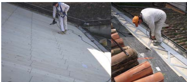
Figure 5: nailings of the wooden planking to the joists and securing the steel perimeter curb.
