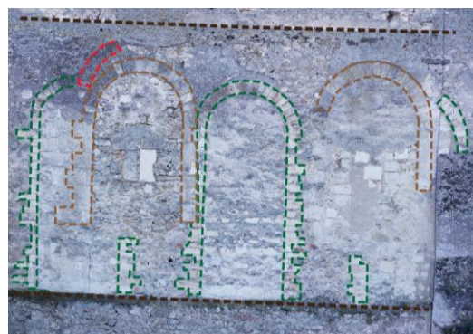
Figure 10 - Projections and plugged windows on the east face of St Paul tower.
