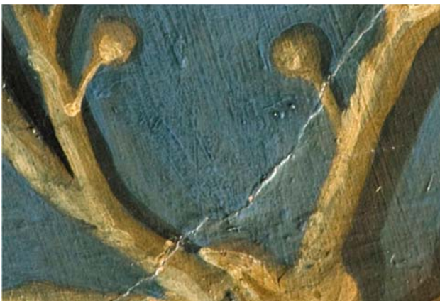
Figure 1. Detail of painted ceiling, taken in 2011, illuminated by raking light, showing an extended crack. The camera was mounted on a tripod at floor level.
